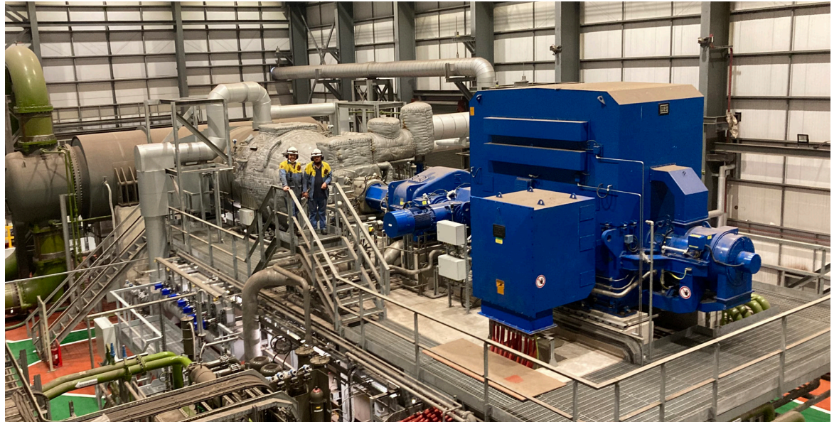
Commissioning Engineer Roger Horton and Power Plant Competency Assessor Darryl Thomas at Port Talbot's new 30MW turbo alternator, which will save money and be better for the environment. The building is also wrapped in Shotton Colorcoat steel
