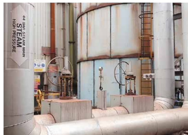
The 44-bar steam main in situ
